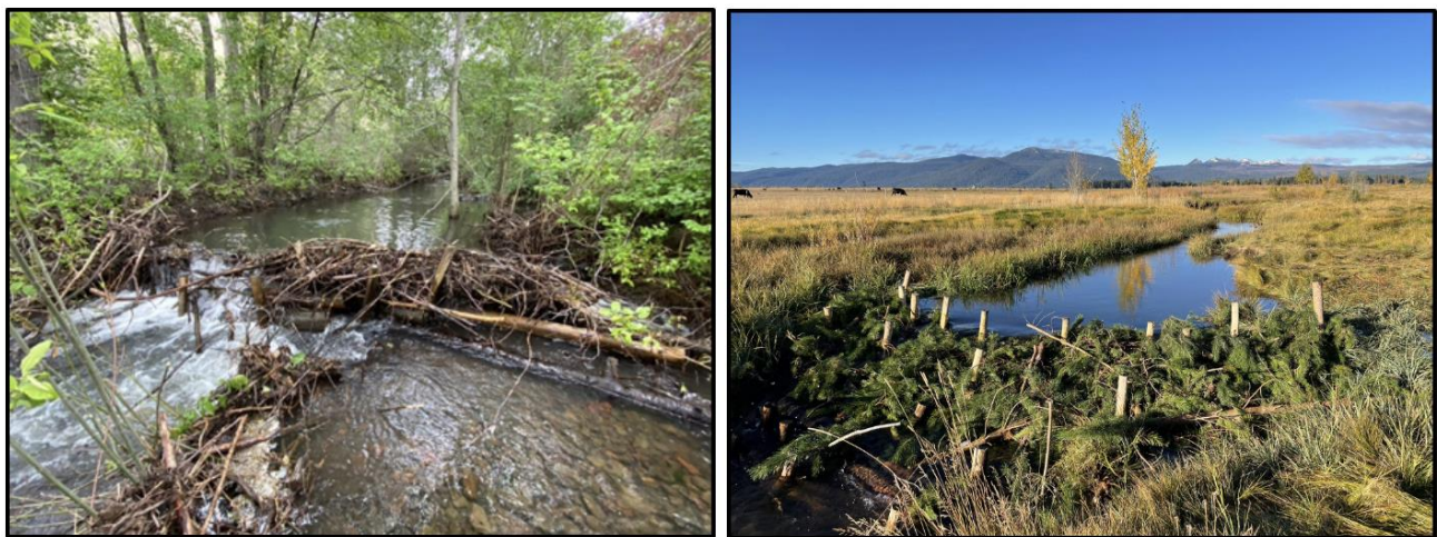
Figure 7: Example of a channel-spanning PALS after multiple years of additional wood accumulation (left photo) and a beaver dam analogue reinforced with posts (right photo).
