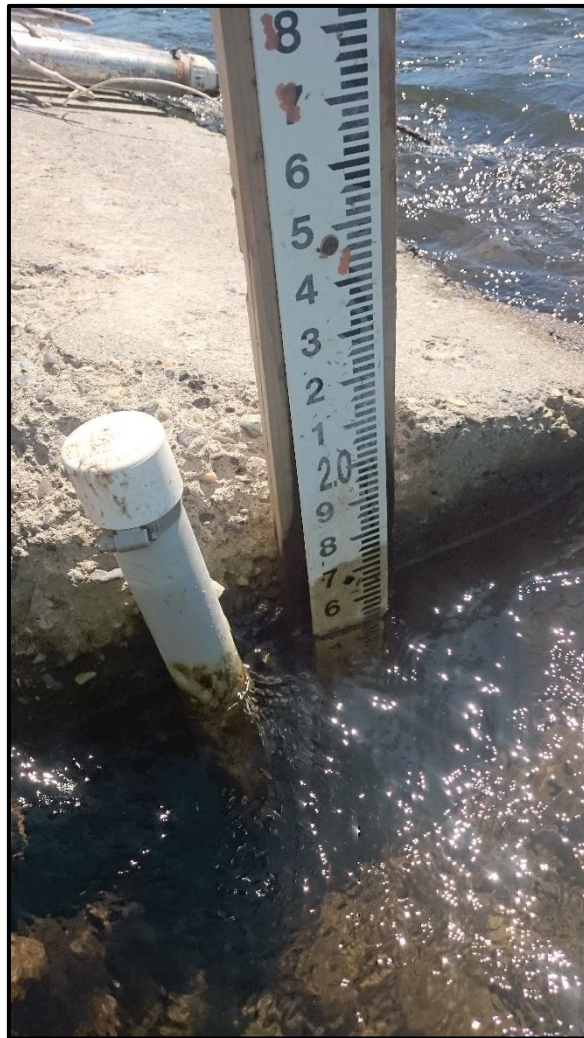
Figure 6. Typical equipment installed at stand-alone monitoring sites that were visited quarterly for manual data download: a staff gauge and perforated PVC stilling well with a suspended pressure transducer.
