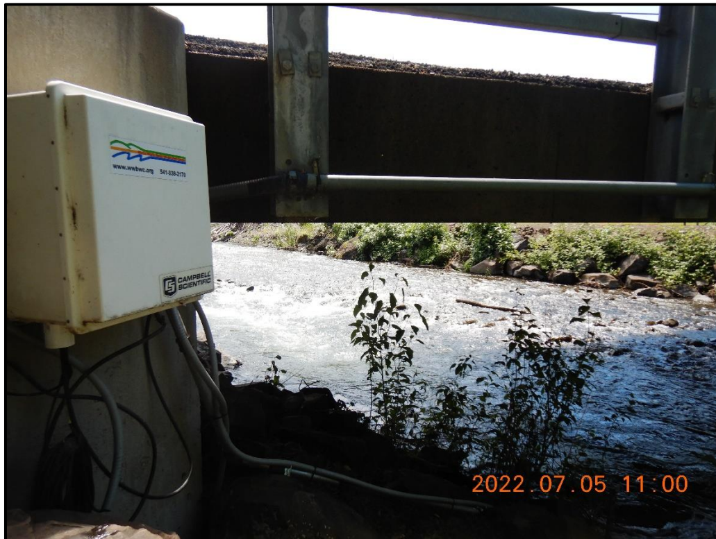
Figure 4. At this near real-time monitoring site on the South Fork Walla Walla River (S-103), a cabled sensor, secured to posts, collects water level data. A communication cable transmits the information to a data logger and radio housed in the gauge box. Using radio telemetry, water level and temperature data are sent to the WWBWC office to be processed and published online.
