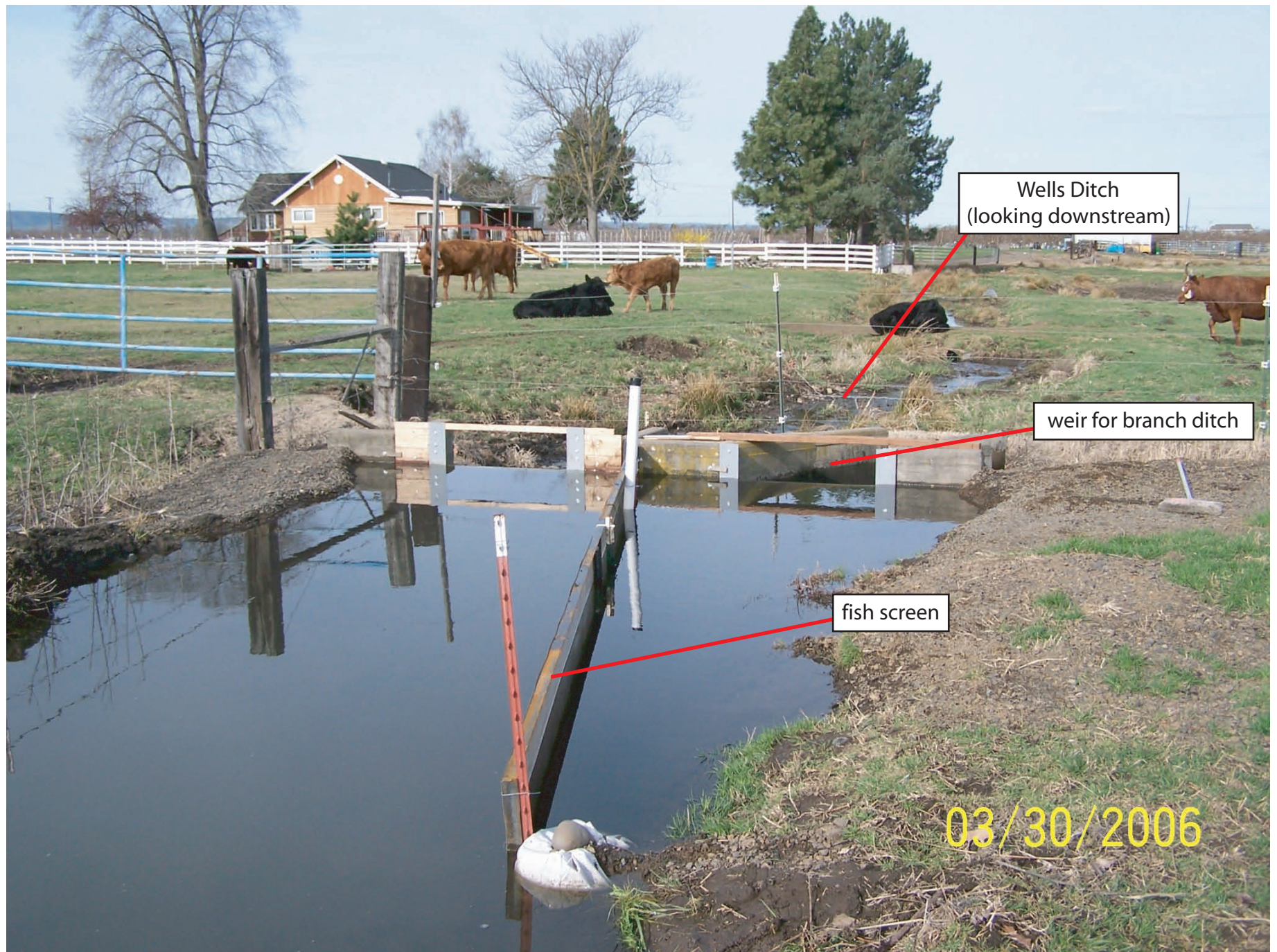
Figure 14. Photograph of the fish screen and weir at the branch ditch diversion off Wells Ditch.
