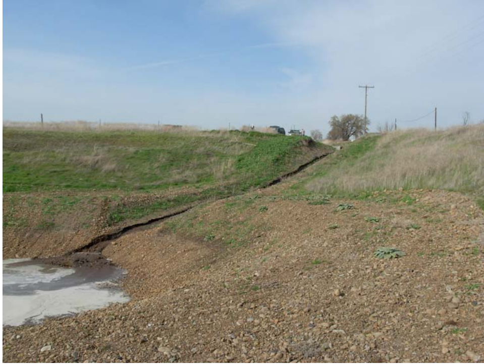
Figure 11. Ditch leading into upper basin. Ramp flume is visible just above head of ditch in background.
