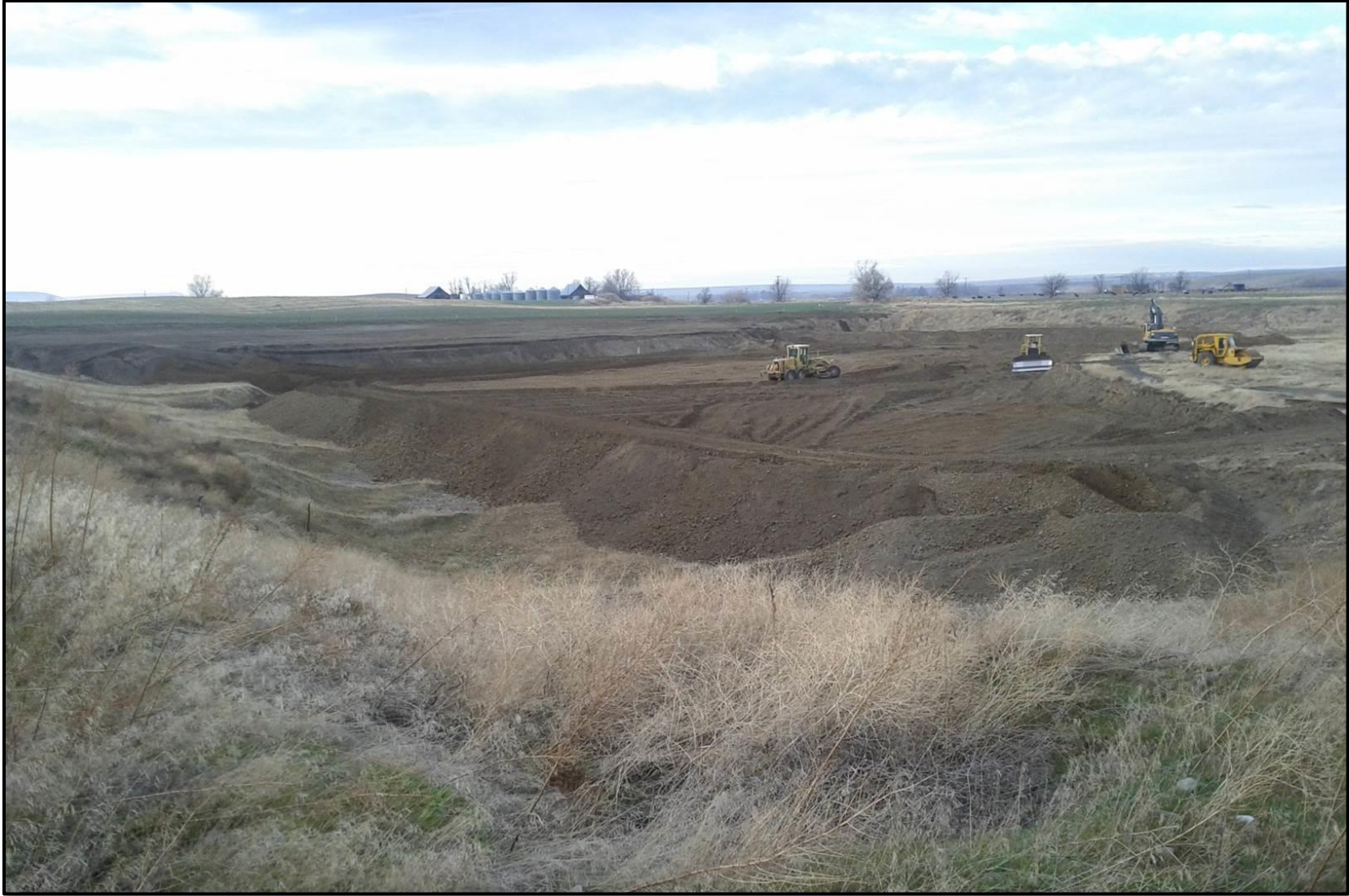
Figure 5- The Locher Road Aquifer Recharge Project during expansion activities in late 2011. The project was expanded from ~1/3 acre basin to a ~2 acre basin. The project basin is located within a historic gravel quarry.
