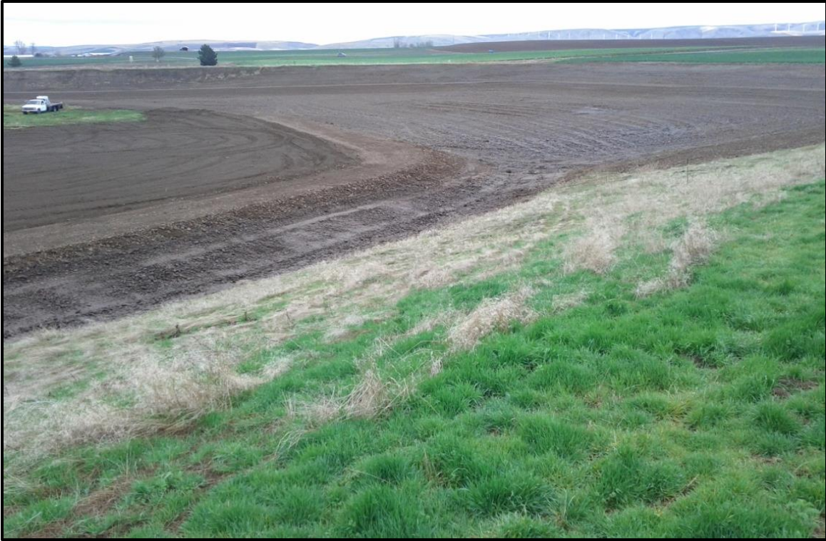
Figure 13 - Photo of the completed expansion of the Locher Road site's main recharge basin, December 2011.
