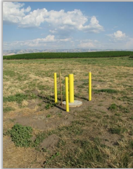
Figure 39. WDOE Funded Dedicated Observation Well at Pepper Bridge Vineyards Road Grange Hall (Washington)
