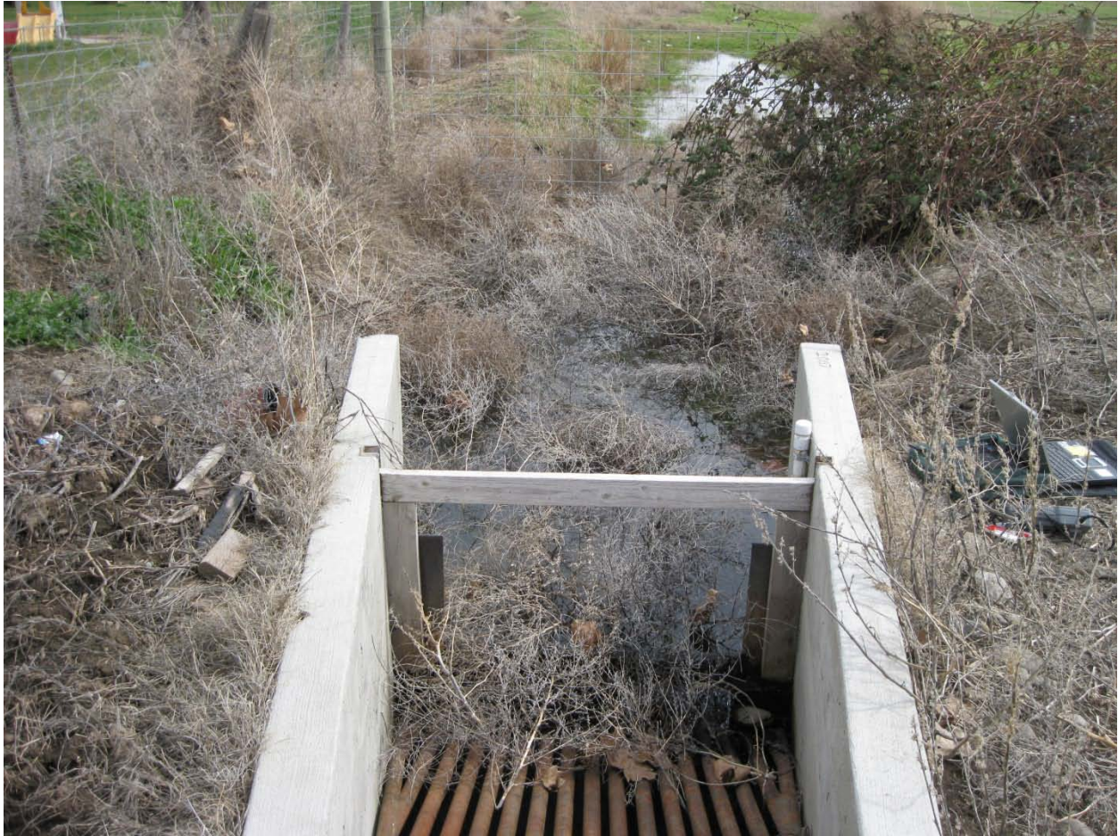
Figure 13. S-410 in Johnson Creek. The creek flows into a pond in a pasture, under the fence shown here, over the sharp-crested weir, and into the metal grate where it flows into a pipe. Tumbleweeds like these seasonally clog up this weir and impede the water's flow.
