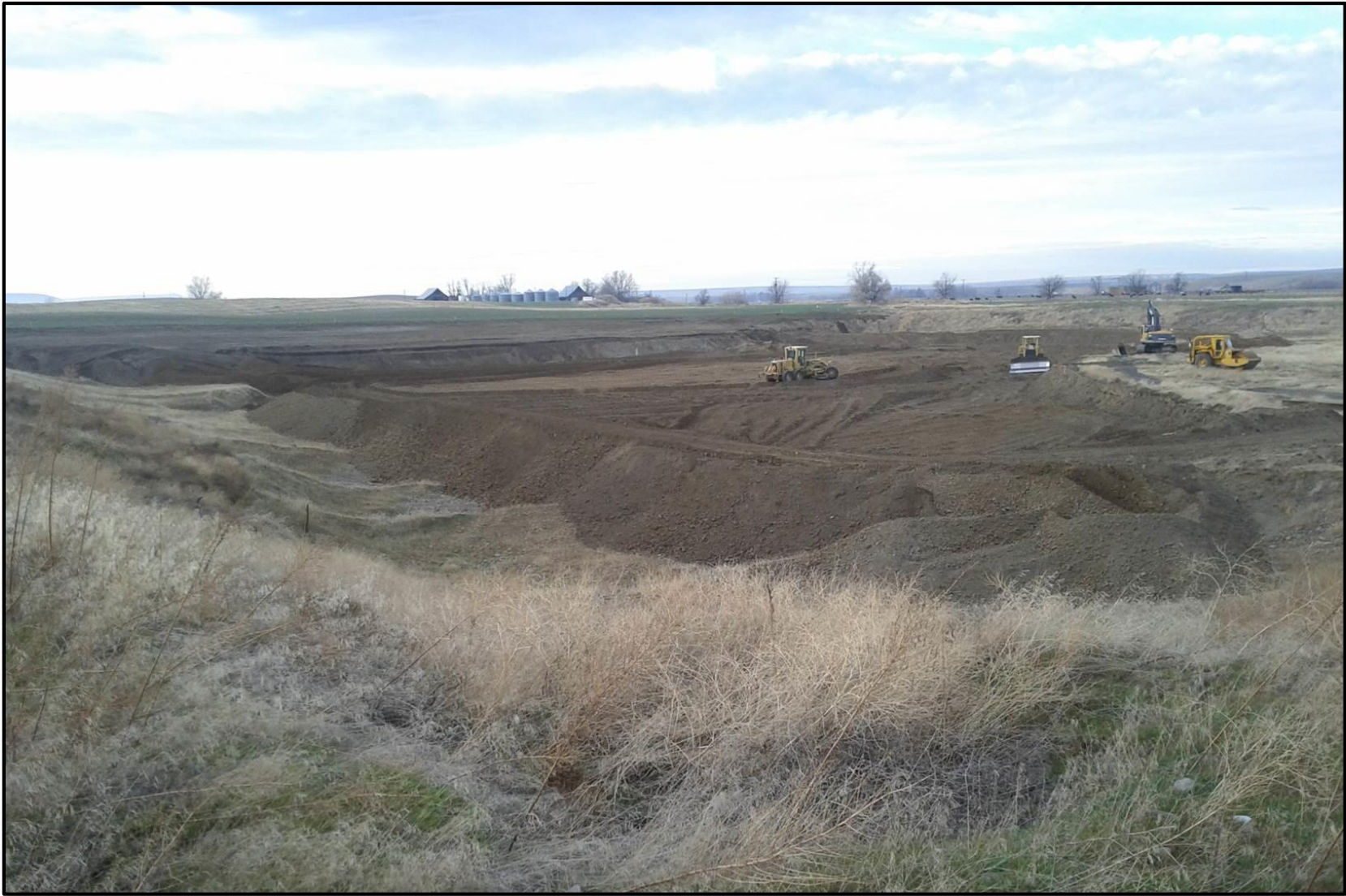
Figure 4- The Locher Road Aquifer Recharge Project during expansion activities in late 2011. The project was expanded from ~1/3 acre basin to a ~2 acre basin. The project basin is located within a historic gravel quarry.
