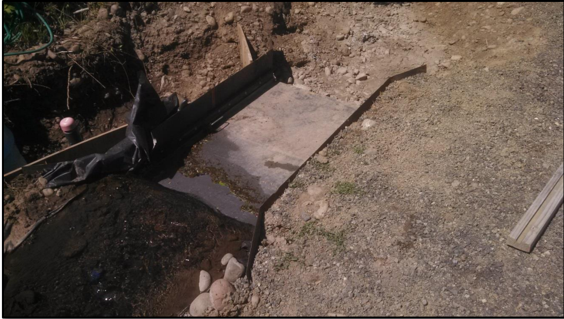
Figure 17 - The turnout structure for the Anspach Aquifer Recharge site. The structure was built by Custom Technology Co. Inc. based in Yakima, WA. The 8" pipe emerges from a flange on the far side of the structure after the water has passed through a 0.062" perforated punch screen. The screen is removable for cleaning purposes. See Appendix D for designs.
