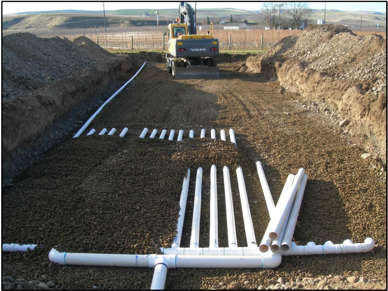
Figure 12 - Photograph of infiltration gallery #2 (IG2) being installed at the Johnson Aquifer Recharge site. IG2 is 4" perforated drain field pipe installed over washed gravel and buried in ~1 foot of washed gravel with geo-textile fabric on top of the gravel. See Appendix D for designs.
