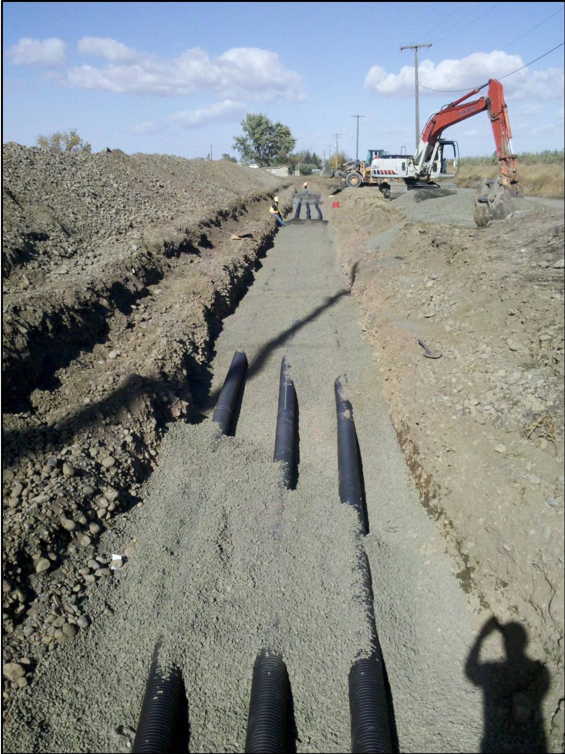
Figure 15 - The Trumbull Aquifer Recharge site under construction in October 2012. This recharge site utilizes 8" perforated pipes instead of the 4" pipes used at the Johnson site. The site is approximately 300 feet long with three 8" pipes running the entire length. See Appendix D for designs.
