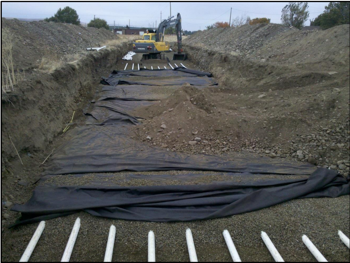
Figure 16 - The Anspach Aquifer Recharge site during construction in October 2012. This recharge site utilizes 10 4" perforated pipes that run approximately 200 feet. See Appendix D for designs.
