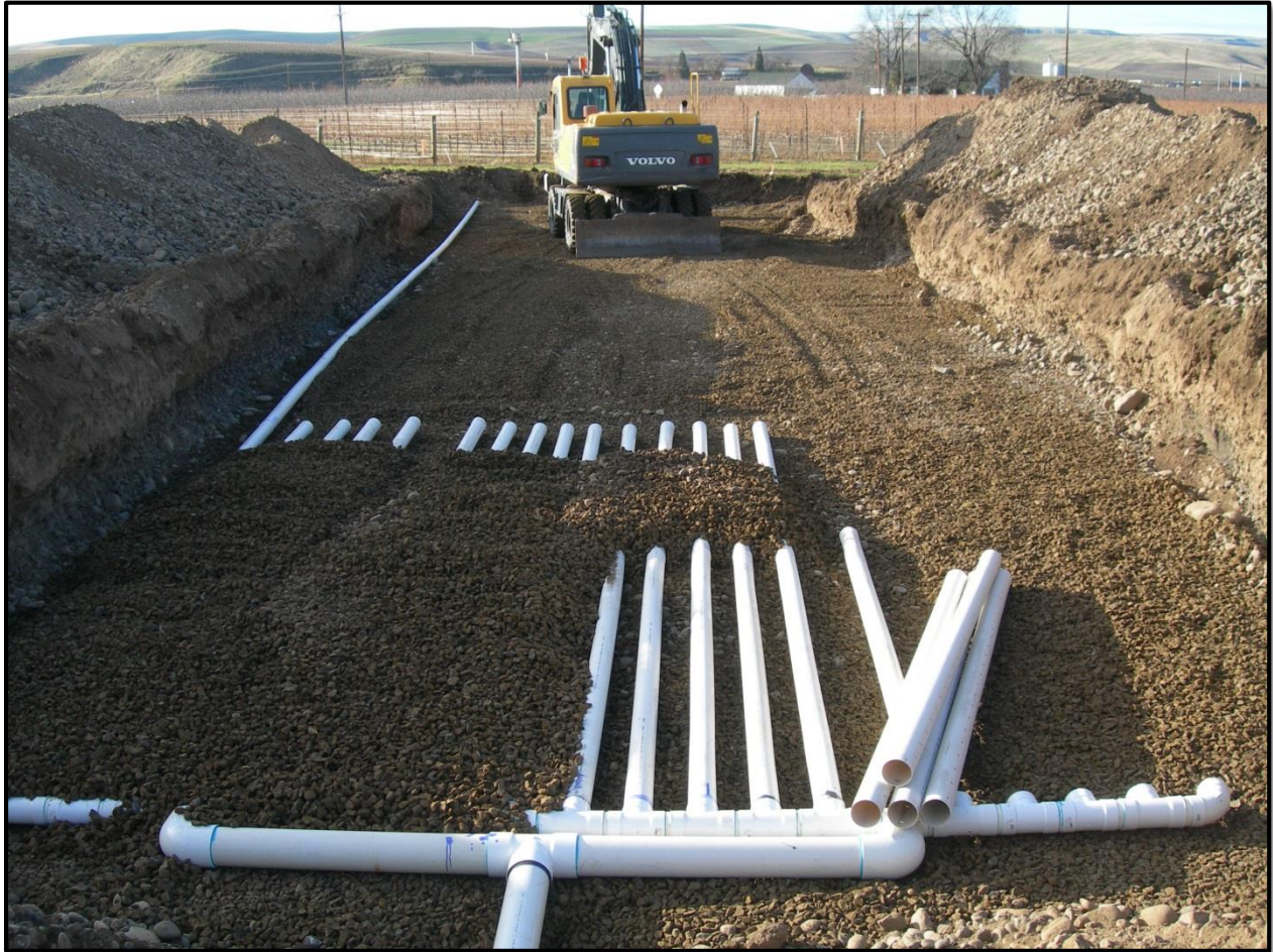
Figure 16 - Photograph of infiltration gallery #2 (IG2) being installed at the Johnson Aquifer Recharge site. IG2 is 4-inch perforated drain field pipe installed over washed gravel and buried in ~1 foot of washed gravel with geo-textile fabric on top of the gravel. See Appendix C for designs.
