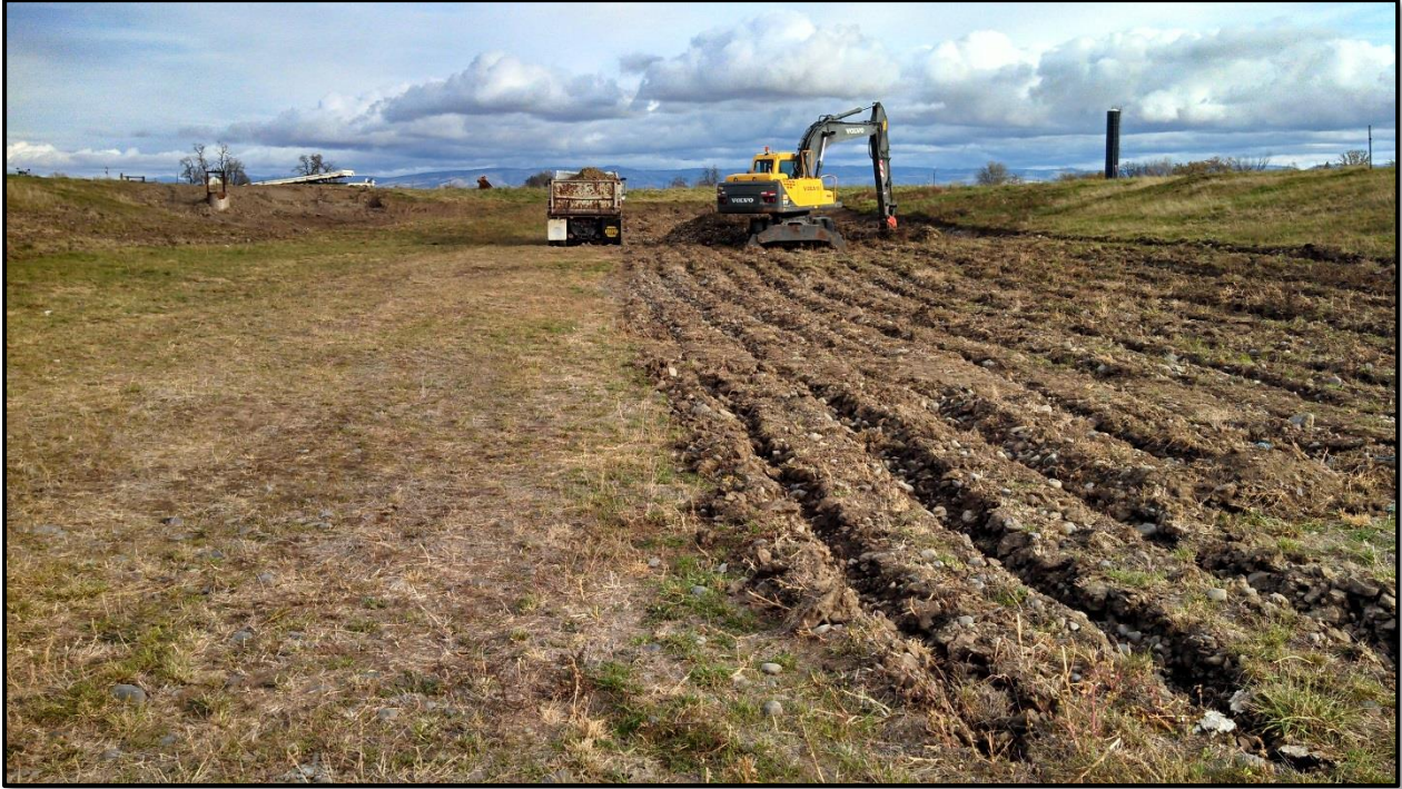
Figure 19 - NW Umapine Aquifer Recharge site during excavation and shaping of the infiltration basin. See Appendix C for design details.
