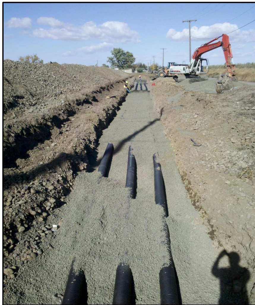
Figure 21 - The Trumbull Aquifer Recharge site under construction in October 2012. The site is approximately 300 feet long with three 8-inch" pipes running the entire length. See Appendix C for designs.
