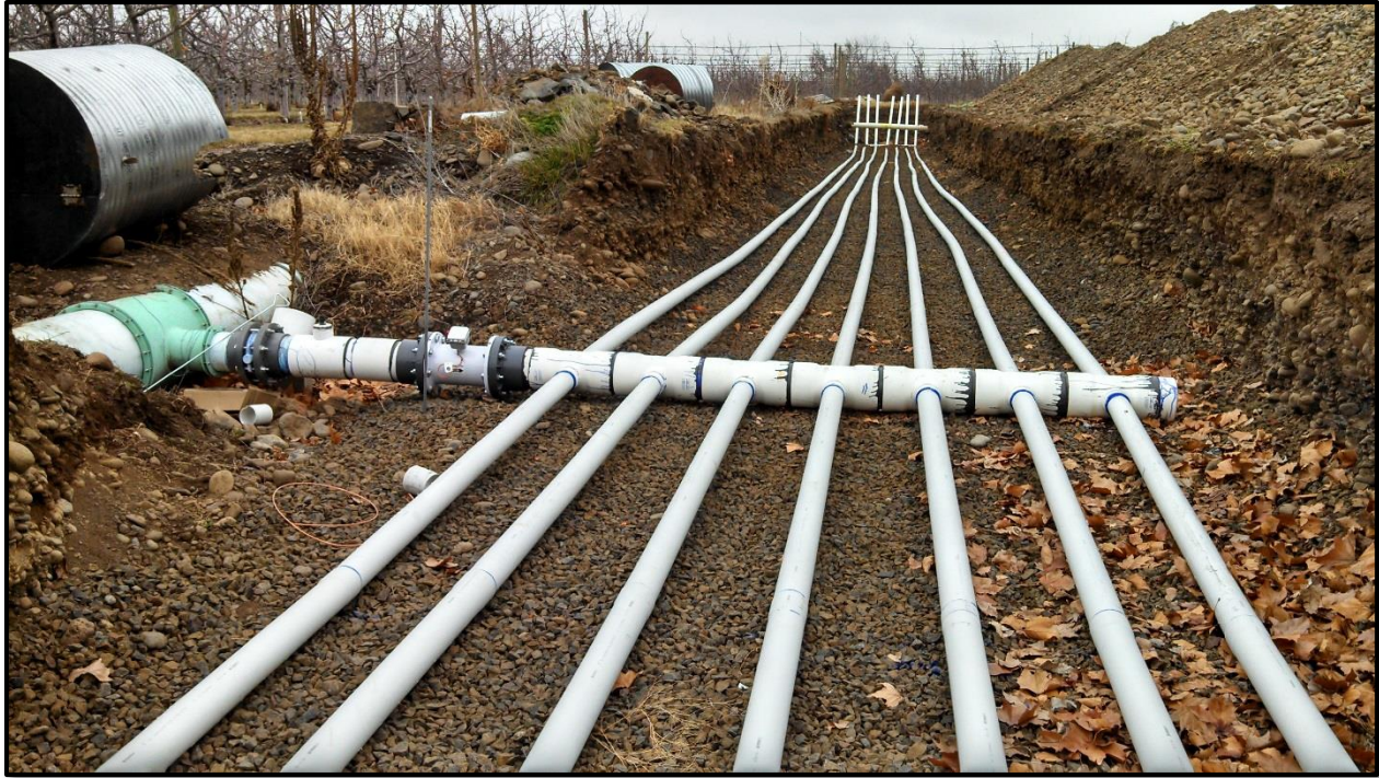
Figure 13 - Turn out structure, flow meter, valve and pipe manifold for the Barrett Aquifer Recharge site. See Appendix C for design details.
