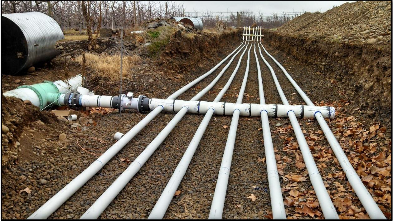
Figure 13 - Turn out structure, valve, flow meter and pipe manifold for the Barrett Aquifer Recharge site. See Appendix C for design details.
