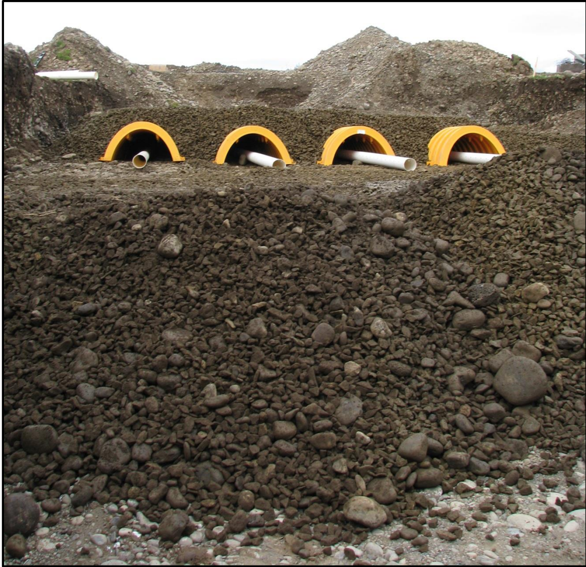
Figure 17 - Photograph of infiltration gallery #3 (IG3) at the Johnson Aquifer Recharge site. IG3 is 4-inch perforated drain field pipe installed within Stormtech stormwater chambers (yellow covers) over washed gravel and buried in ~2 foot of washed gravel with geo-textile fabric on top of the gravel. See Appendix C for designs.
