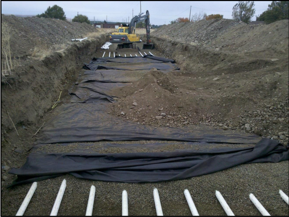
Figure 10 - The Anspach Aquifer Recharge site during construction in October 2012. This recharge site utilizes 10 4-inch perforated pipes that run approximately 200 feet. See Appendix C for designs.
