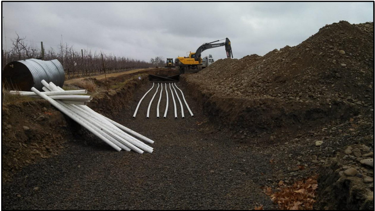
Figure 12 - The Barrett Aquifer Recharge site during construction in January 2014. This recharge site utilizes 7 4-inch perforated pipes that run approximately 600 feet. See Appendix C for designs.
