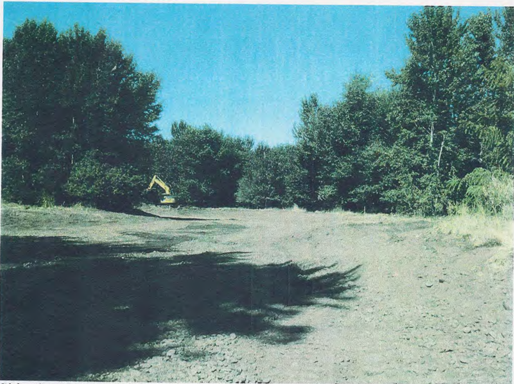
Side channel area is being excavated. Existing vegetation was planted in late 1990s
