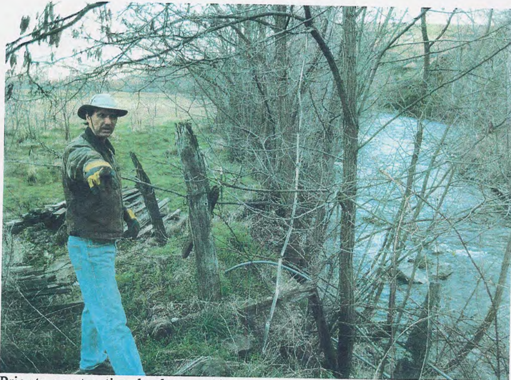
Prior to construction, landowner Clark Lampson stands on edge of eroding riverbank where damaged levee will be removed as part of project, about a 10' drop to water
