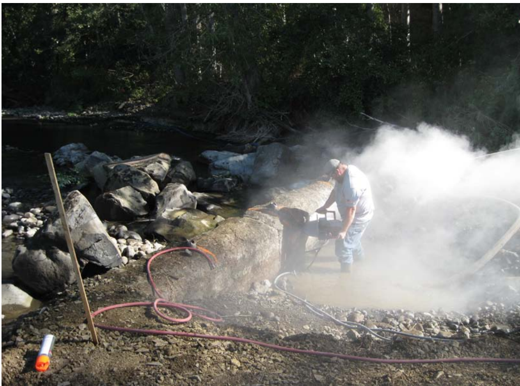
This photo shows a technician from A-Core, Inc. completing the concrete cutting.
